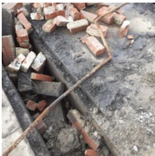
Plate 1: Hydrocarbon staining on surface at location of a former substation on site.
